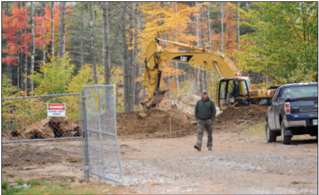
Pete Hamilton, superintendent for Gary Chicoine Construction, said Tuesday they are getting as much done as possible before the ground freezes at the senior housing project in Conway. (JAMIE GEMMITI PHOTO)
